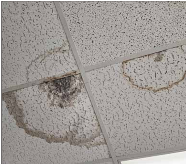
SOME CEILING PANELS AT JUNCTION WERE STAINED, AS DOCUMENTED BY PARENTS IN A REPORT TO THE DISTRICT DATED MARCH 26.
