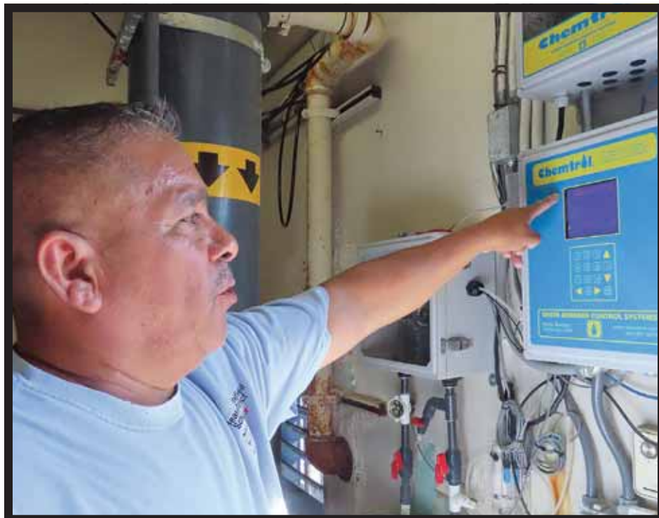
Leal goes over the control system that shows him the different chemical levels for the pool at Foothill, which he checks at least twice a day.
