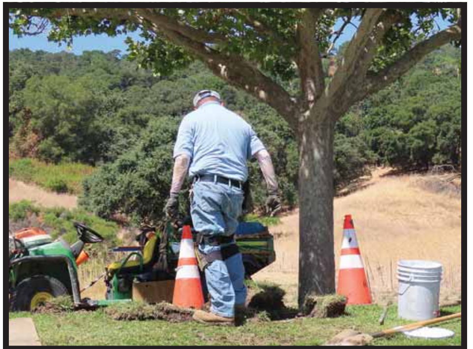
Foothill's groundskeeper works on fixing the school's main pipe on Aug. 7, which Leal said had been leaking. Leal said the groundskeeper had to take the whole pipe apart and put it all back together before school started the following day.
