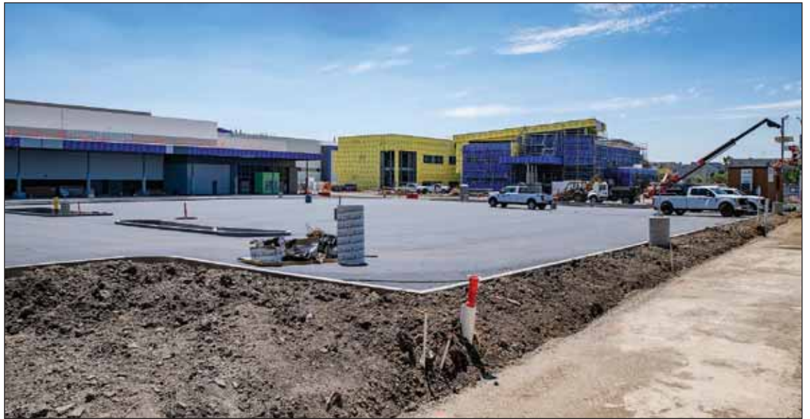
Construction progress at the site of Emerald High School, which will be Dublin Unified School District's second comprehensive high school.
