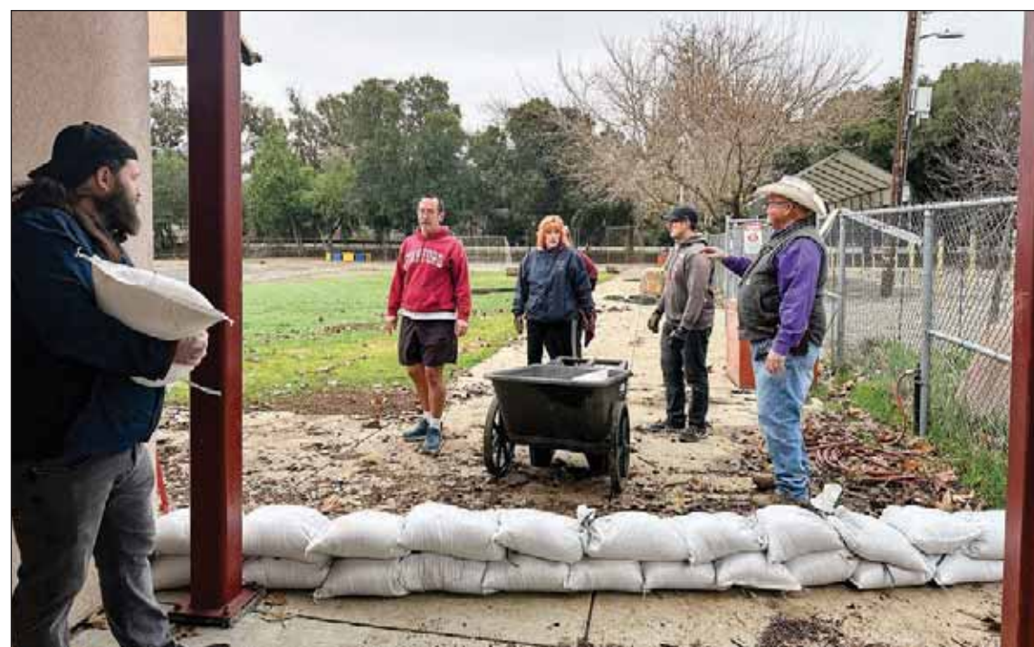
Sunol Glen School staff work on cleaning up the school after the New Year's Eve storm and place sand bags in preparations for last week's additional storms.
