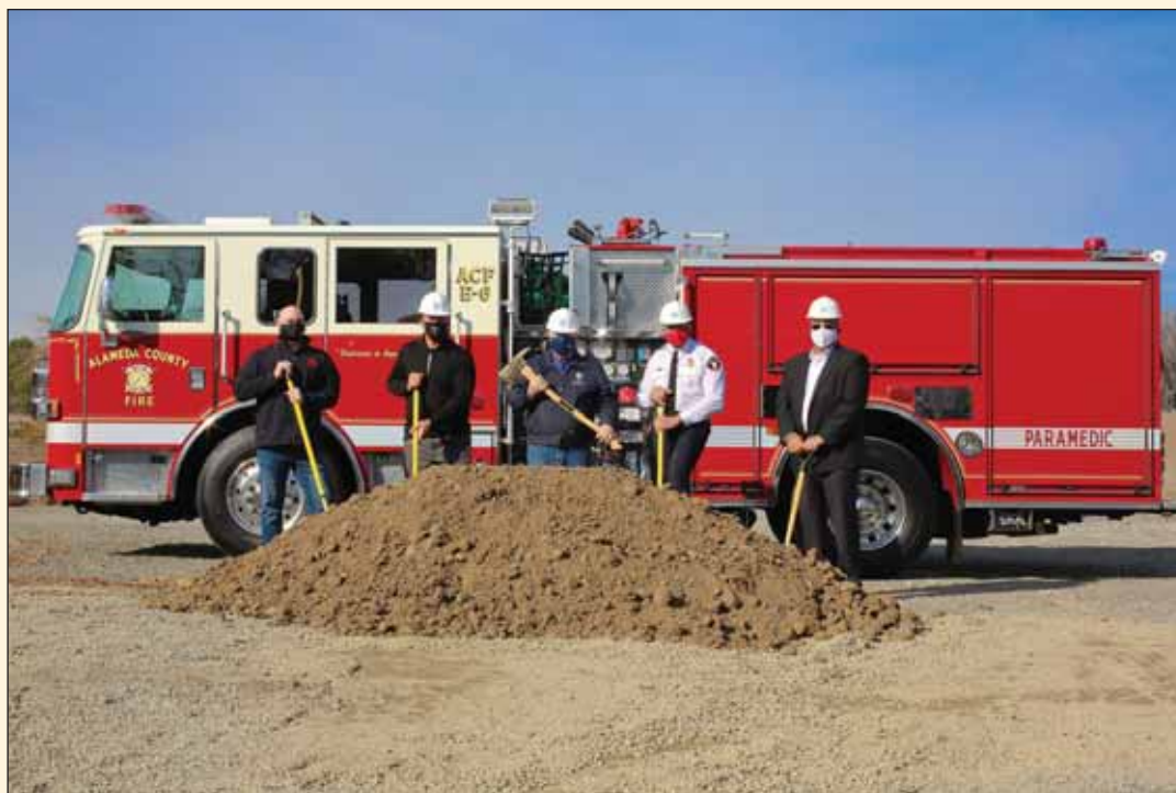
Alameda County officials, including outgoing Supervisor Scott Haggerty (center), attend the ceremonial groundbreaking of the new ACFD Regional Training Center in Dublin.
