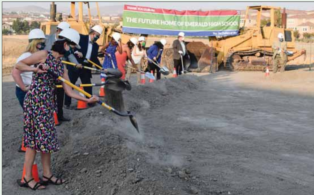
Dublin officials, shovels in hand, turn the dirt during the groundbreaking ceremony Sept. 30 at the site of the future Emerald High School.
