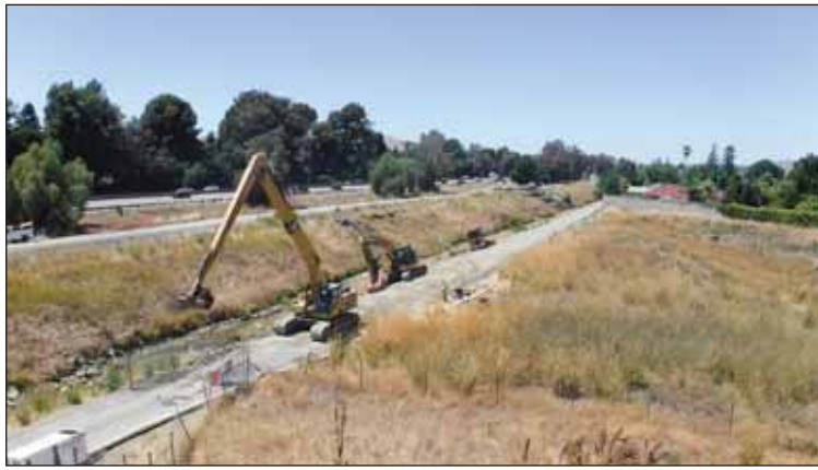
A stretch of the Centennial Trail in Pleasanton was reopened on July 26 after repairs to an adjacent flood control channel were recently completed.
