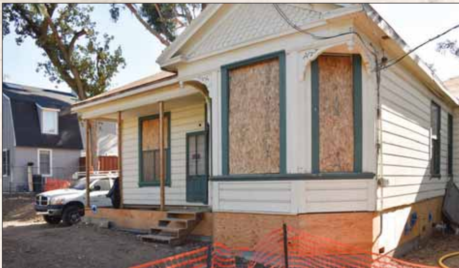
The house at 309 Neal St. is currently in the midst of renovations, though the new owners are required to keep the building's exterior, as visible from the front, in its original historical form.
