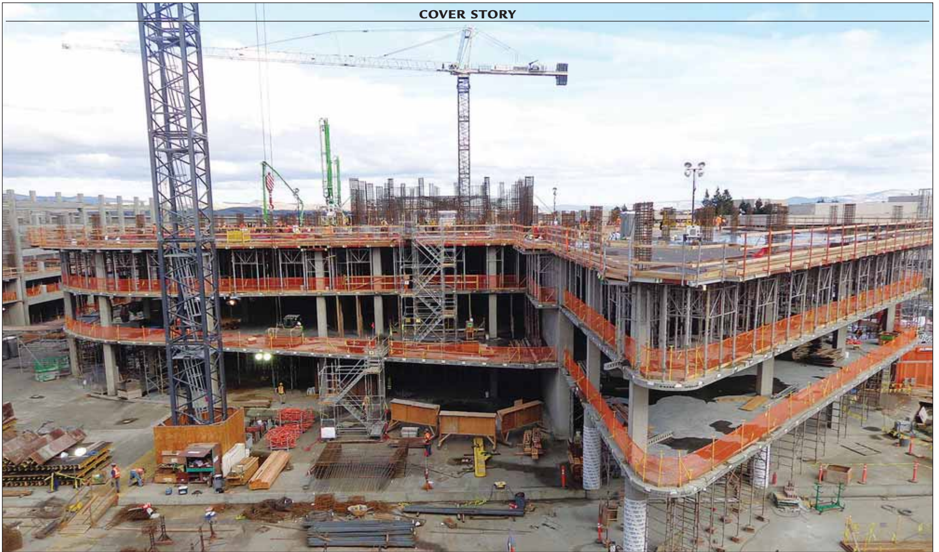
Work continues on first three floors of Workday's new six-story corporate headquarters building under construction on Stoneridge Mall Road. The facility will be completed in early 2019.
