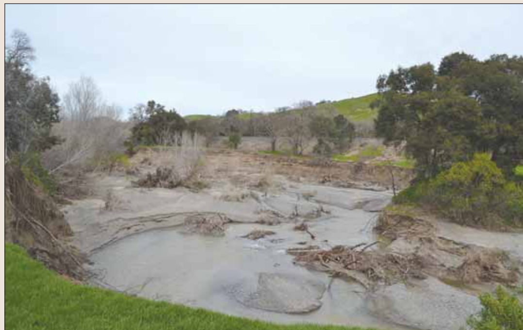
An s-turn that has developed in the Arroyo de la Laguna is directing water toward multiple Foothill Road homes and eroding their backyards. JULIA REIS
