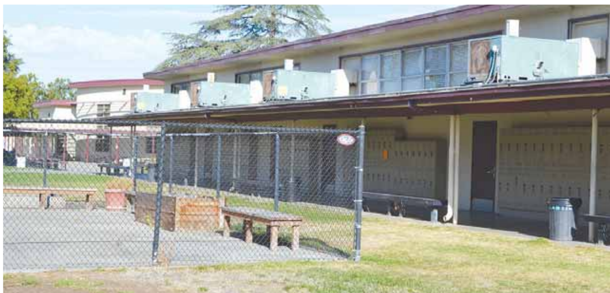
District officials say the HVAC systems district-wide, like these at Amador Valley High School, are outdated.
