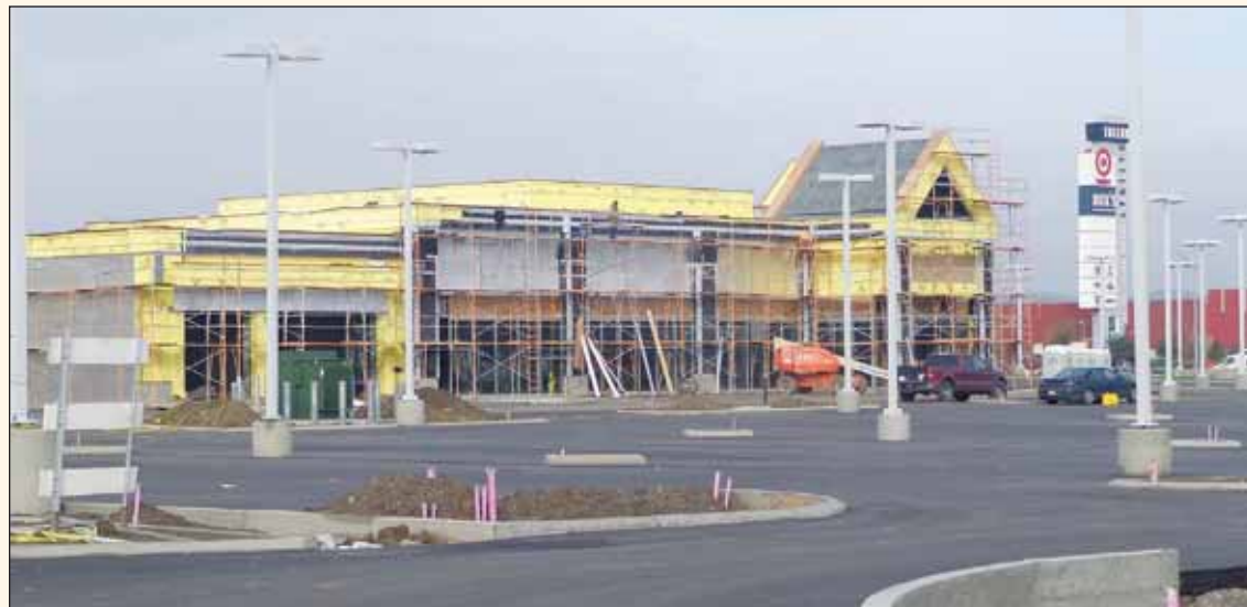
Construction work continues on CarMax superstore in Staples Ranch off I-580 near El Charro interchange. CarMax, the country's largest retailer of used cars, will open locally this spring.
