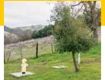
Hydrant connection already in place since 2003 — 210' from Sunset Creek Lane
