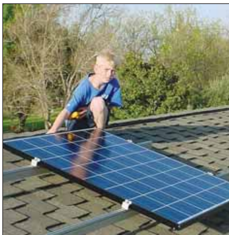
Chris Spooner, who was 10 when this picture was taken, helps install solar panels. Both he and his older brother Jason helped in the installation, which was all done by the Spooner family.
