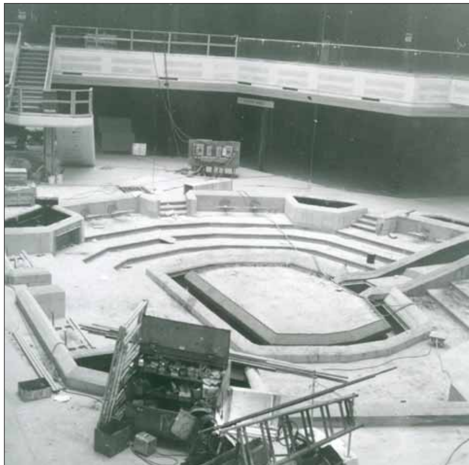
Grand Court in center of Stoneridge Shopping Center under construction in late 1979
