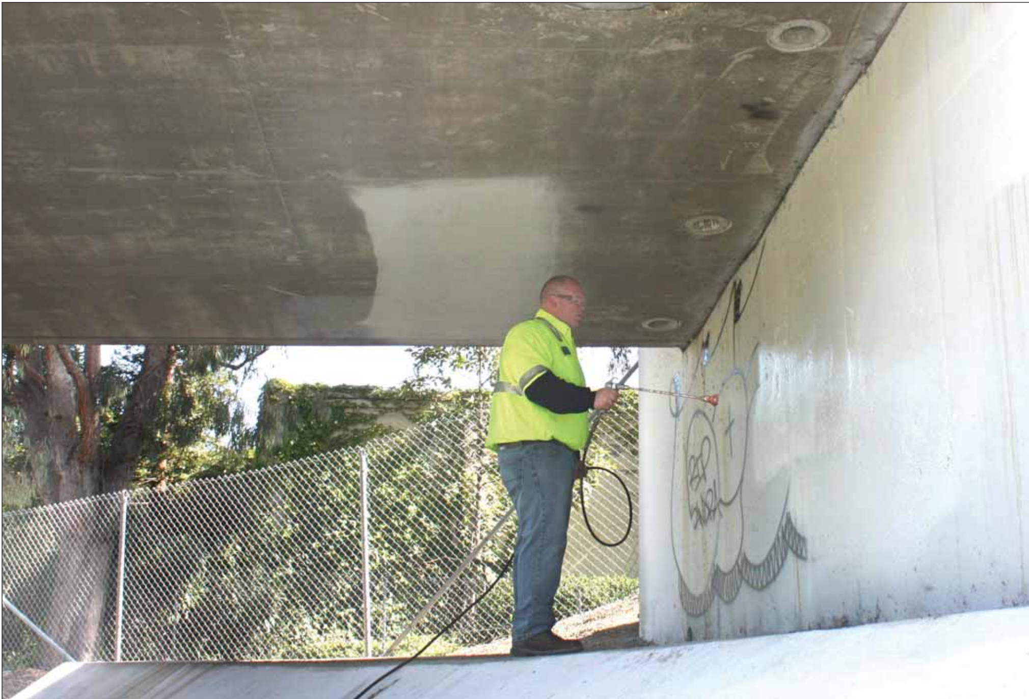
Sam Morris, a maintenance worker for the city of Pleasanton, uses an airless spray rig, the same rig used to paint curbs, stripe streets and parking lots, to cover up fresh graffiti along the Alamo Canal Trail last Friday.
