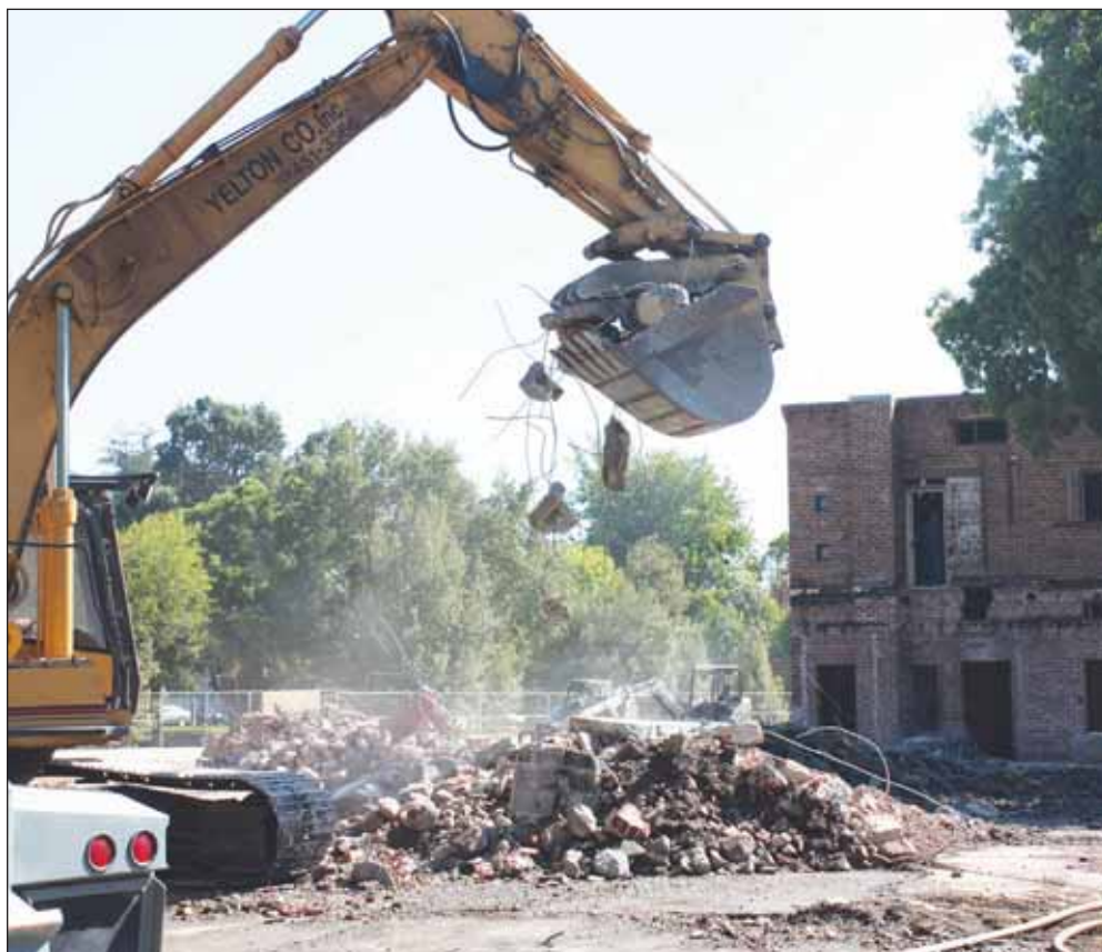
A wrecking crew dug into portions of the old fire stations No. 1 and 4 on Railroad Avenue in the fall, in preparation for the Firehouse Arts Center, which will open early 2010.
