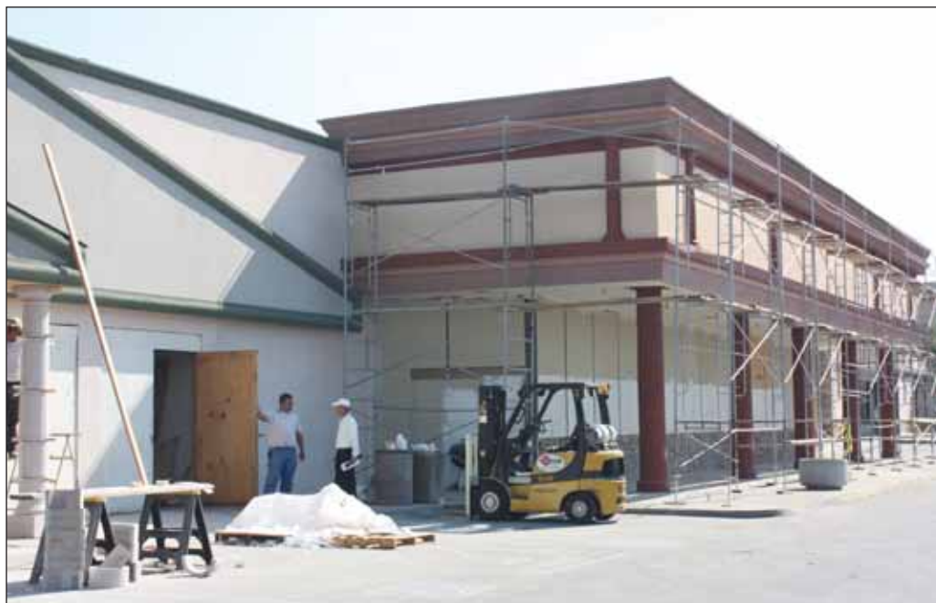
Construction manager Jose Hernandez, at left, said the shopping center is almost finished and landscaping will be planted soon.
