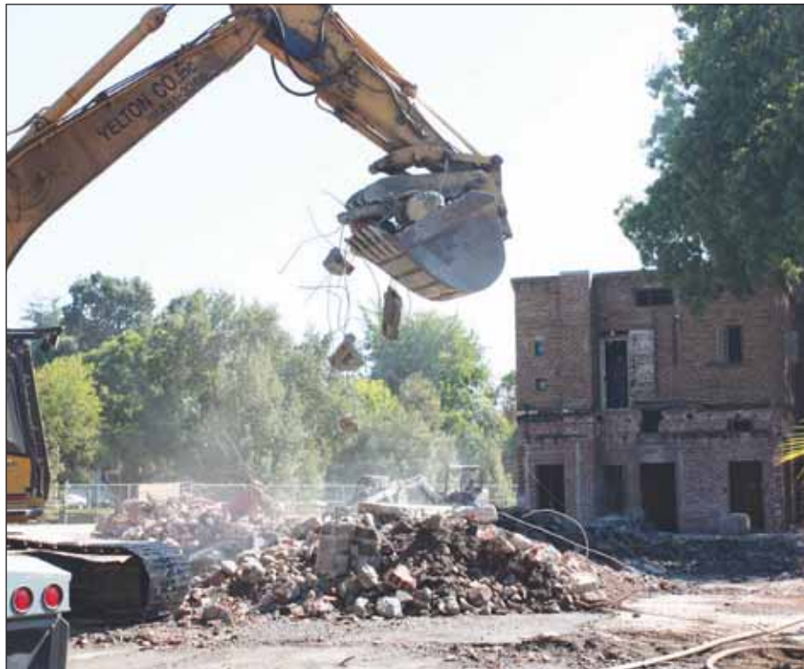
Construction crews dig into the brick of the historic Fire Station No. 1 as they prepare for the restoration of the old firehouse, to be transformed into the Firehouse Arts Center, opening late 2009.
