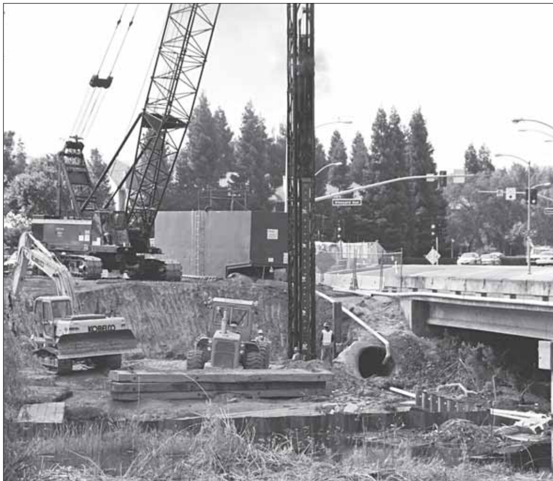
Bulldozers and cranes are hard at work to construct a second bridge over Arroyo Del Valle.
