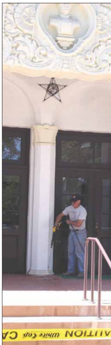
The Veterans Memorial Building on Main Street was reopened in November after a $4.5-million restoration.
