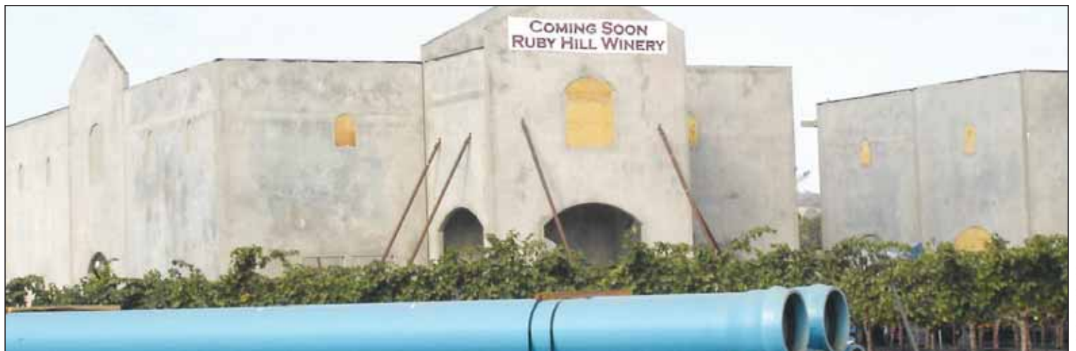
Large blue pipes lie at the future front entrance of the Ruby Hill Winery, located at the corner of Vineyard and Isabel avenues on Pleasanton's southeastern border with Livermore.
