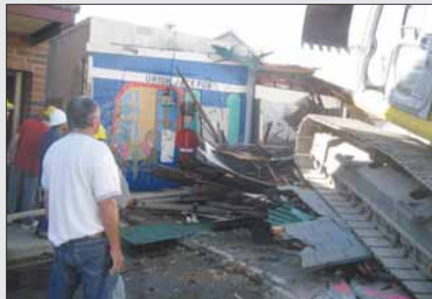
A wrecker's claws dig into the 1880s-era building, making short work of the once-famous downtown bar.
