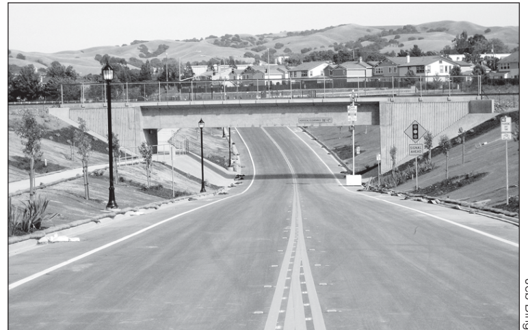
All paved, striped and ready for cars, this new $5.3-million underpass for Valley Avenue below the Union Pacific Railroad tracks seems to flood due to heavier ground seepage than expected. Its opening will await installation of back-up pumps that are now on order.
