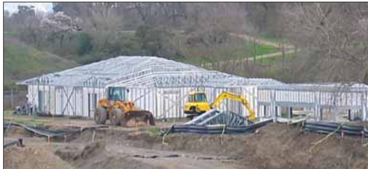
Although scheduled to be completed and open by Memorial Day 2005, a walk-through of the Splash Waterpark at Shadow Cliffs Regional Park shows only some progress in the construction of the steel framework for a future food concession, ticket sales office and an administration building.
