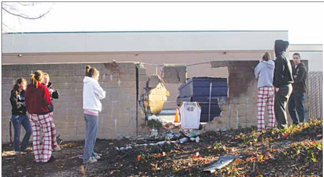
Friends of 16-year-old Kyle "K.O." O'Connor gathered Wednesday morning at the crash site where there's now a gaping hole in a cinderblock wall behind the DMV in the 3600 block of West Las Positas Boulevard.
