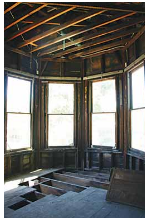
Exposed and damaged flooring, overhead rafters and window frames under the Kolln Building cupola await replacement with custom-milled materials that will exactly replicate the original materials.
