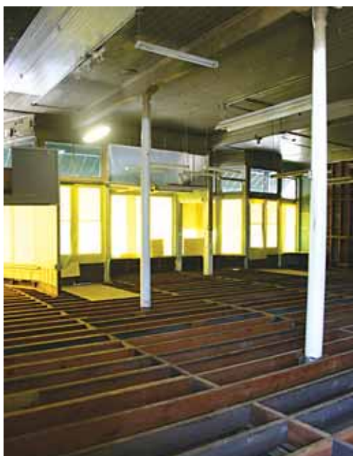
Floor joists, many of them redwood, show up in this photo after the plywood floor was removed. Like the symmetrically-milled white wood support posts, they sit on dirt, seen since Kolln Hardware was built in 1898.
