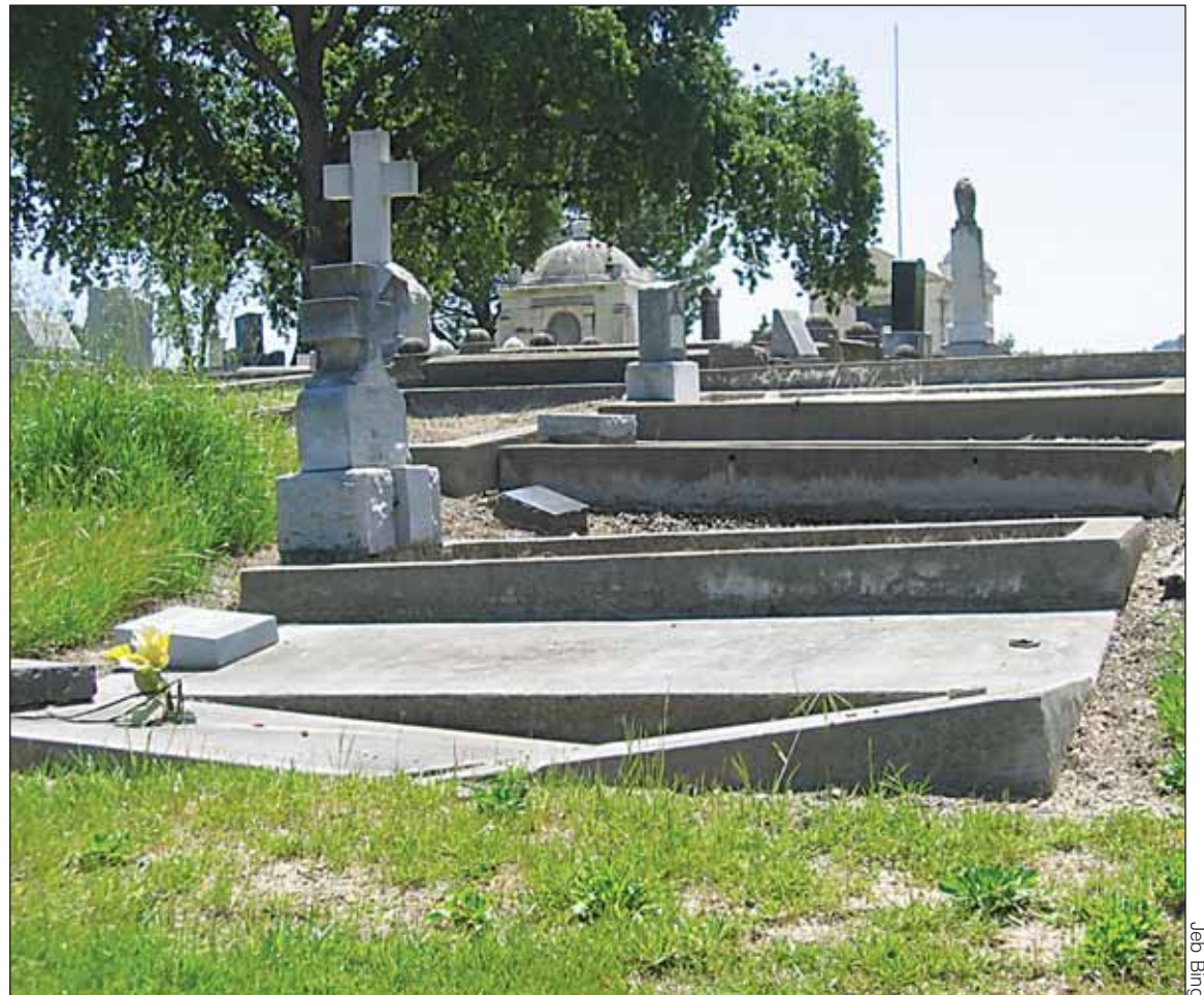
Cracked, sinking and deteriorating old grave markers such as this one are found in about half of Pleasanton Memorial Gardens, which the Livermore Odd Fellows lodge wants to sell to Pleasanton. So far, the City Council, seeing the repairs costs, has said no.
