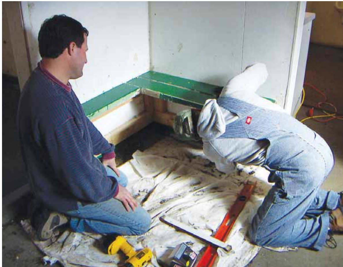
Tim Buteau (left) and Frank Gouveia help fix the restrooms at Camp Loma Mar during last year's renovation project.
